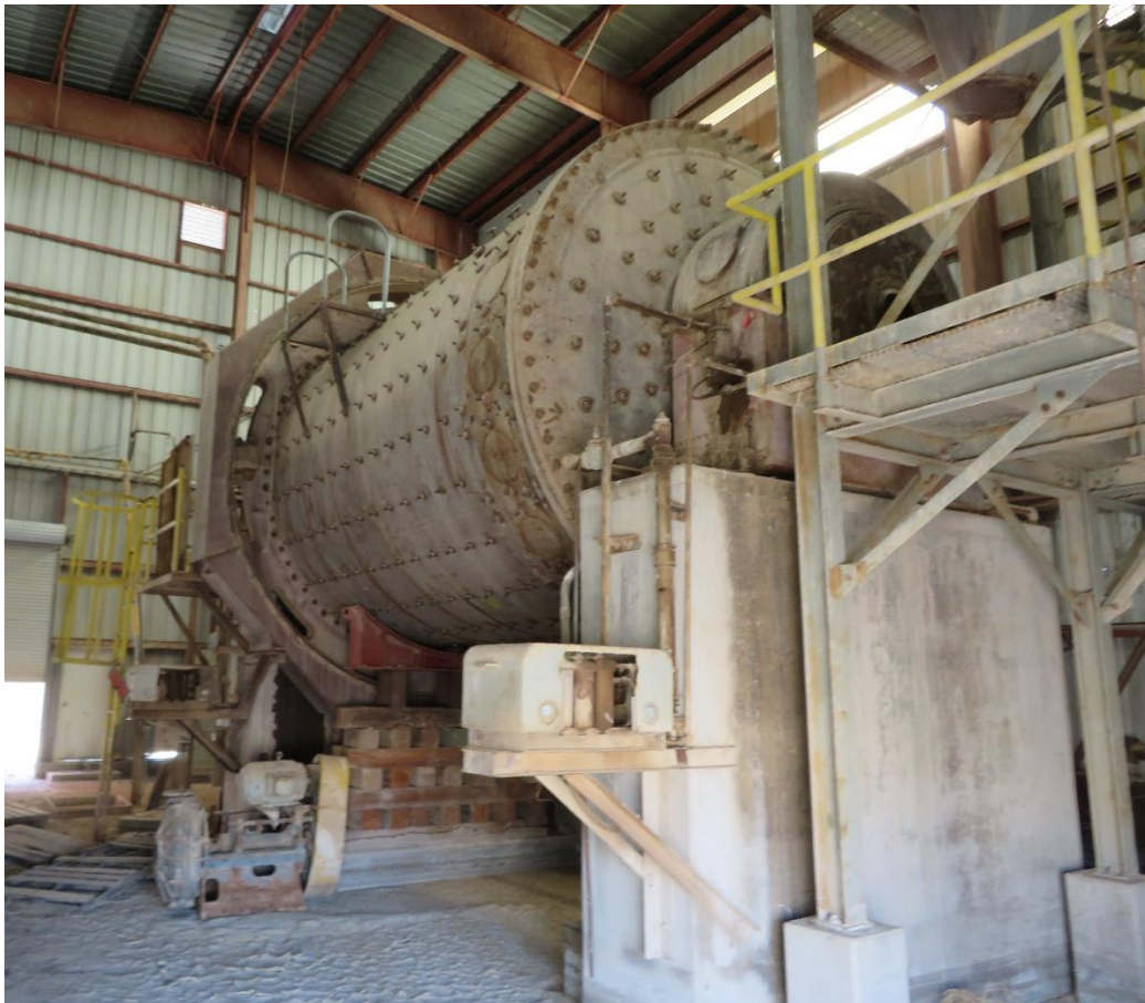
Photo: Ball Mill inside Mill Building
